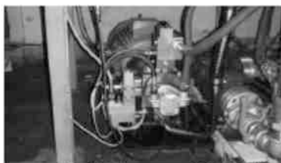
Fig. 10. Servo pump MOOG within the primary sector of hydrostatic transmission.
