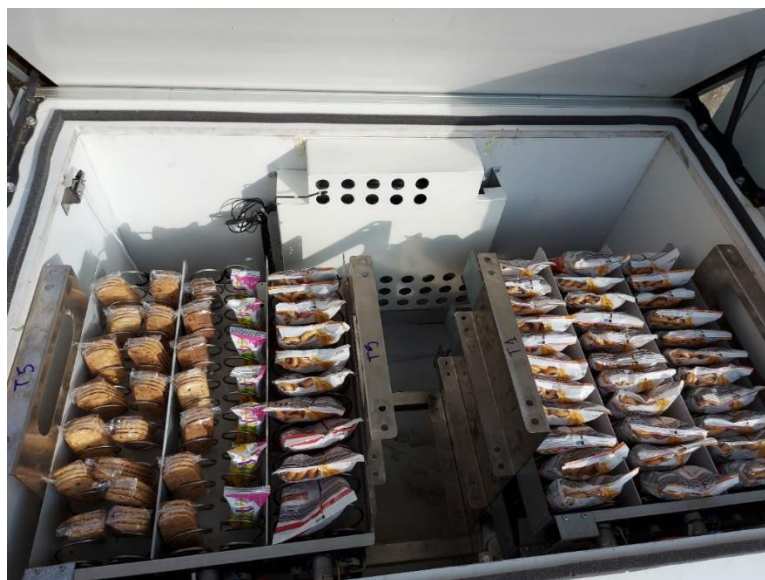
Fig. 7. Thermally insulated enclosure
