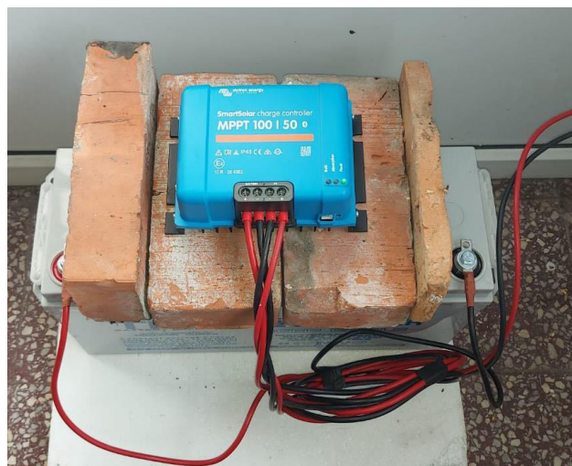
Fig. 11. MPPT charge controller
