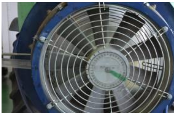
Fig. 2. Determining the speed of air from behind the fan
