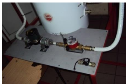
Fig. 6. Hot water circulation electro-pump
